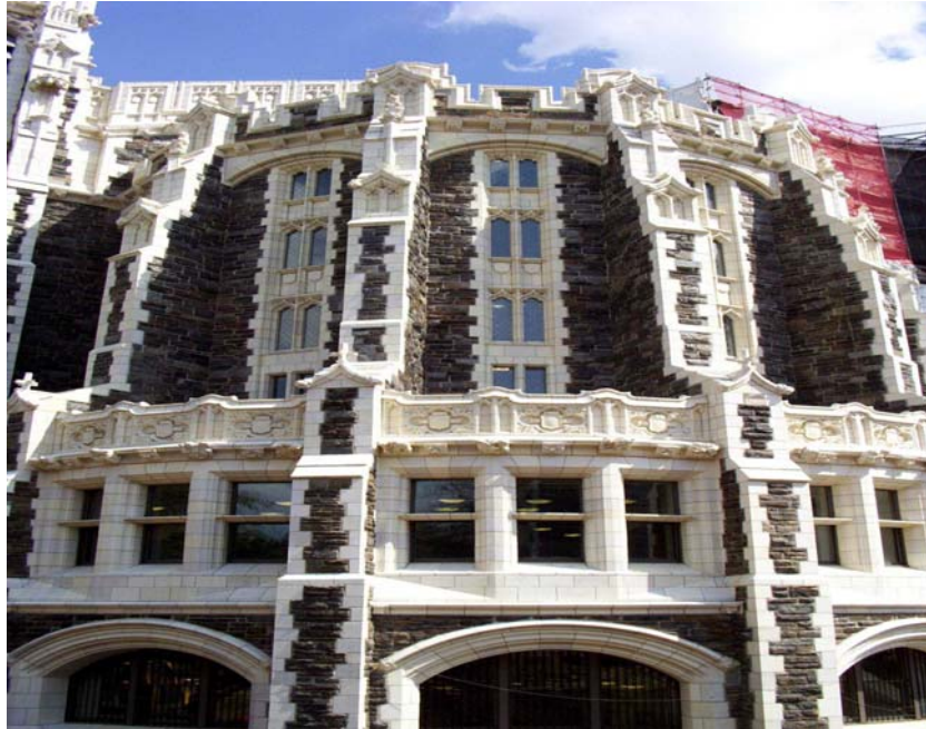
Fig 11 Terra Cotta Replacement on Shepard Hall, New York - 72000 units with more than 4000 shapes inc.sculptures
