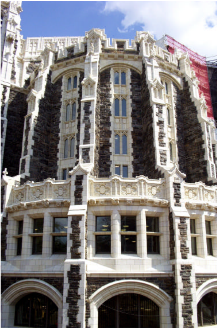
Figure 5: The reconstruction of the exterior of Shepard Hall, built in 1907, is a multi-phase project that will eventually lead to the replacement of 72,000 units and over 4000 shapes, including many ornate sculptures. The project is still on-going and it is a tribute to GRC that many of the new elements are being fixed next to 10-year-old pieces with no discernable differences being visible.
