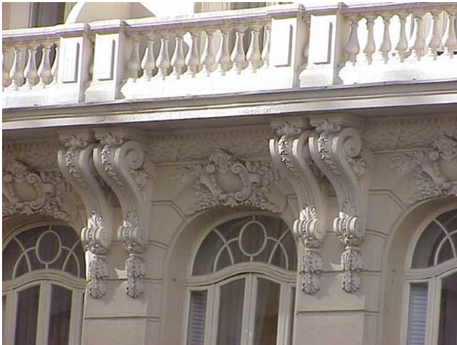
Fig 3 “The highly ornate exterior of the prestigious Palace Hotel in the centre of Madrid, Spain was spectacularly restored to its former glory with the moulded GRC parts being almost indistinguishable from the original carved stone in appearance and texture”
